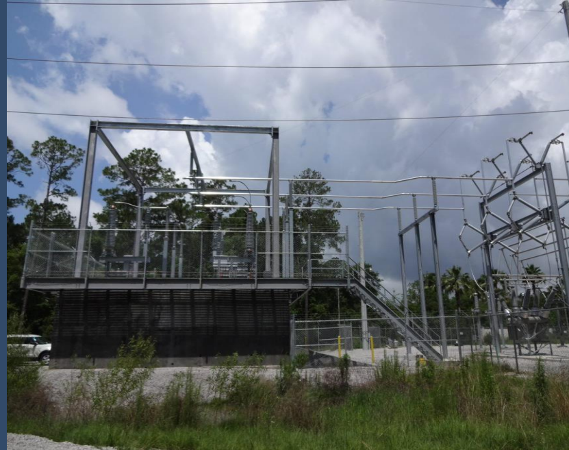
115 kV termination structure for ICWW crossing in Alabama
