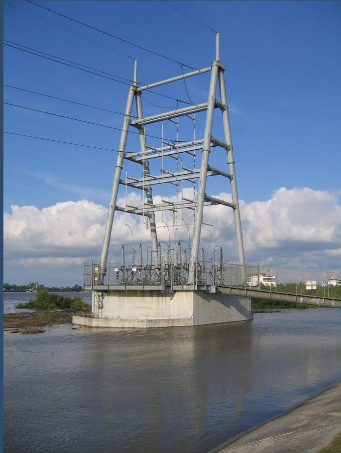
230kV termination structure for Miss River crossing in New Orleans
