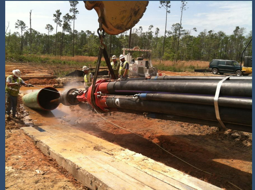
HDD cable bundle (115kV) under Intracoastal waterway in Alabama
