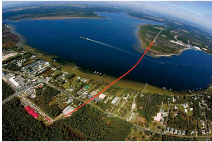
World Record Breaking Directionally Drilled High Voltage Cable Crossing Designed By NELSON
