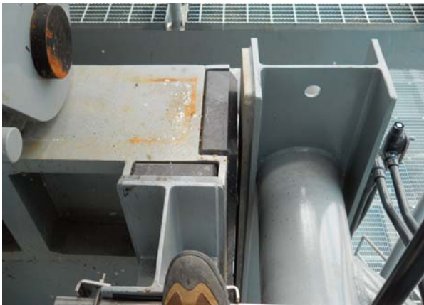
Half Inch Clearance
