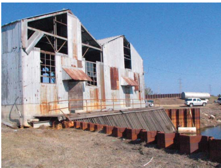
Pump Station Damage
