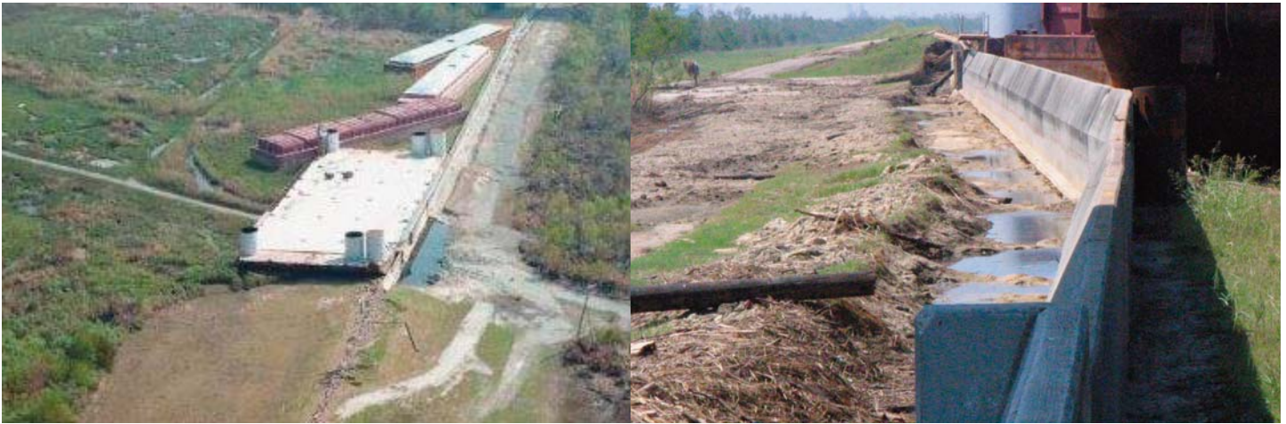
Barge Overtopping Damage to IHNC Floodwall and Levee
