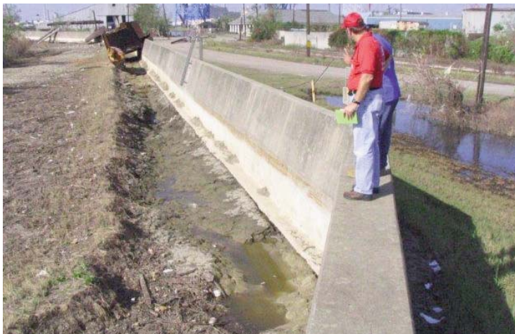
IHNC Floodwall Overtopping Damage
