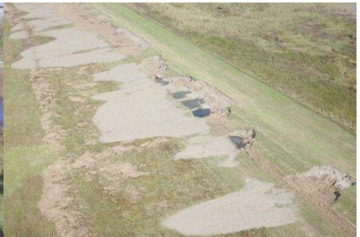
MRGO Levee Damage
