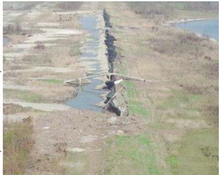
MRGO Overtopping Damage
