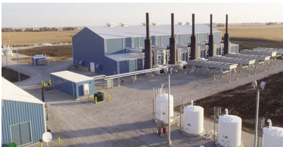
Typical Compressor Station
