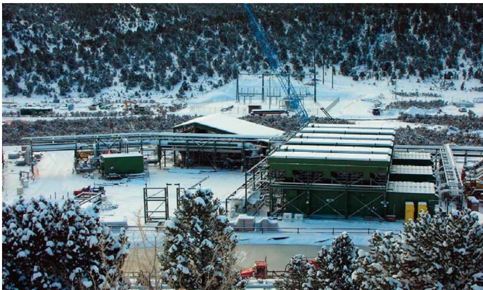
Shell Colorado Freeze Wall Test Facility
