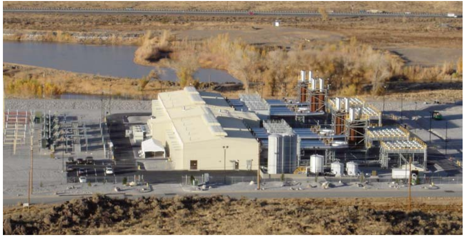
Wärtsilä Barrick Gold Mine Western 102 Power Plant
