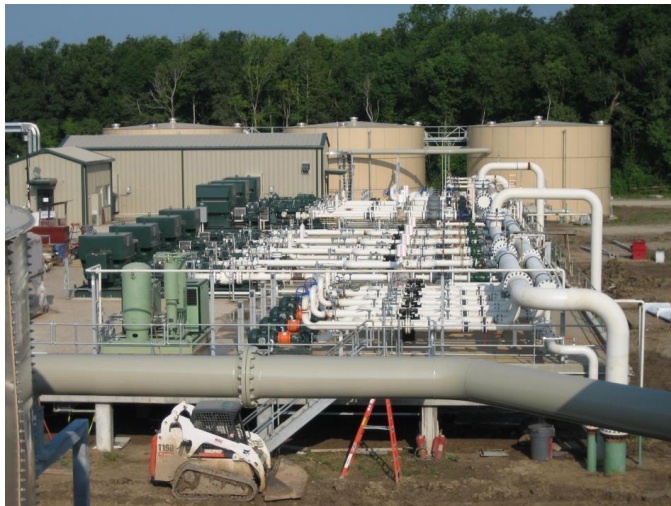
Bobcat Gas Storage Leaching Facility Port Barre, LA Pumping Facilities
